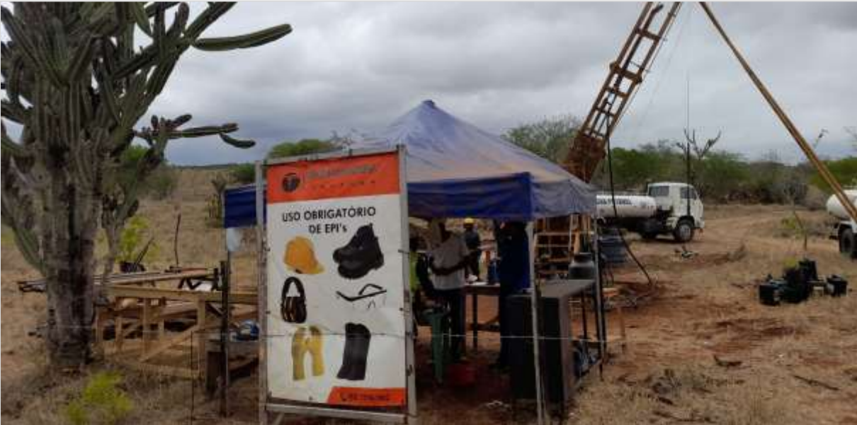
Figure 9.5 All Diamond drilling enclosures are fenced off with appropriate PPE signage on the Capim Grosso Project (Source: QP).
